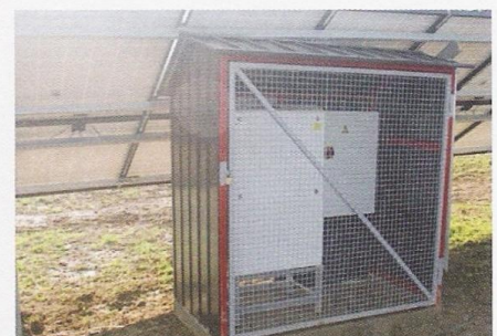
Weatherproof: The inverters of the SolarMax S series can be installed inside and out – even for this freestanding system in Gornji Petrovci.
