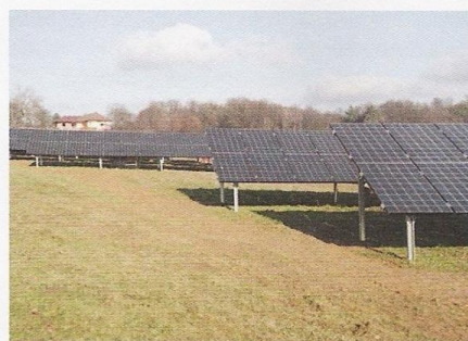
The largest freestanding system in the region: This solar plant in north-slovenian Gornji Petrovci has a power output of 81 kilowatts.
