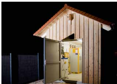
High-tech wooden hayrick: Three Solar Max inverters transform the solar electricity of this megawatt station into grid-compliant alternating current.
