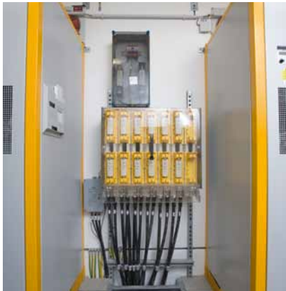
The SolarMax inverters feed their electricity directly into the medium-voltage grid.
