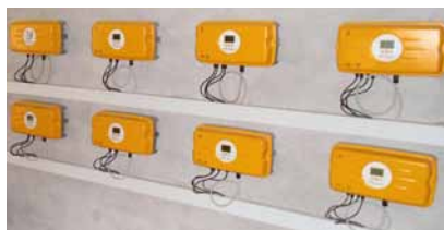
Pin-point precise: The MPP trackers of 16 SolarMax string inverters find the maximum power point for every module string of this PV plant in Altomünster.
