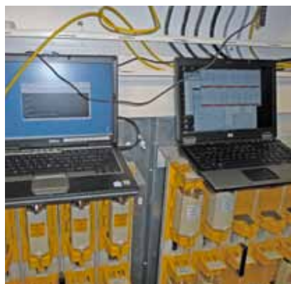
Recorded completely: When the plant was commissioned, Sputnik’s service technicians recorded all the data from the pilot plant.
