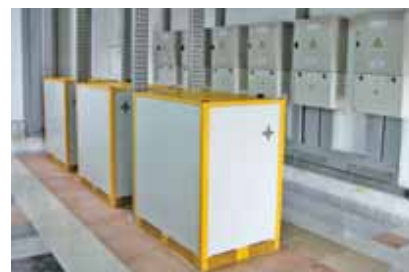
Three SolarMax central inverters transform the current of the largest PV plant on the Canary islands into grid-compliant alternating current.
